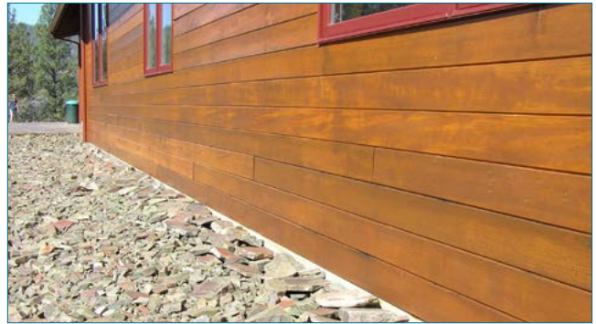
Photo: Stephen Fitzgerald, © Oregon State University Maintain a noncombustible area around the base of your home.
