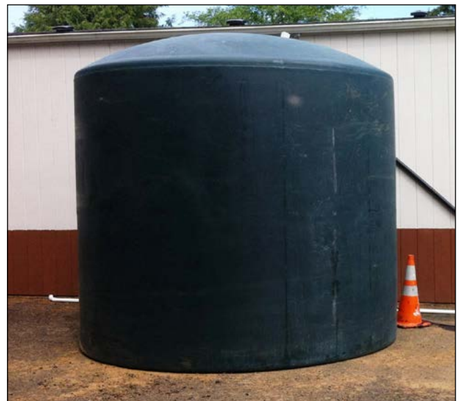
Figure 12. Polypropylene water storage tank with a 10,000-gallon capacity.
