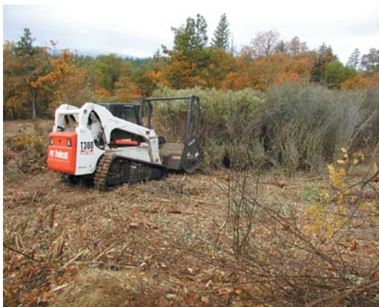
Figure 4. Brush Mulcher treating manzanita and wedgeleaf ceanothus brushfield in southwest Oregon. The cutting head, here mounted on a Bobcat-type tracked vehicle, efficiently cuts material up to 4 inches in diameter. Photo: Paul Howell.
